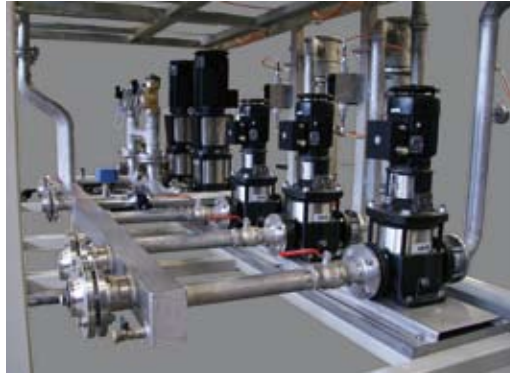
Tubing of the user circuits (secondary circuits) in stainless steel
